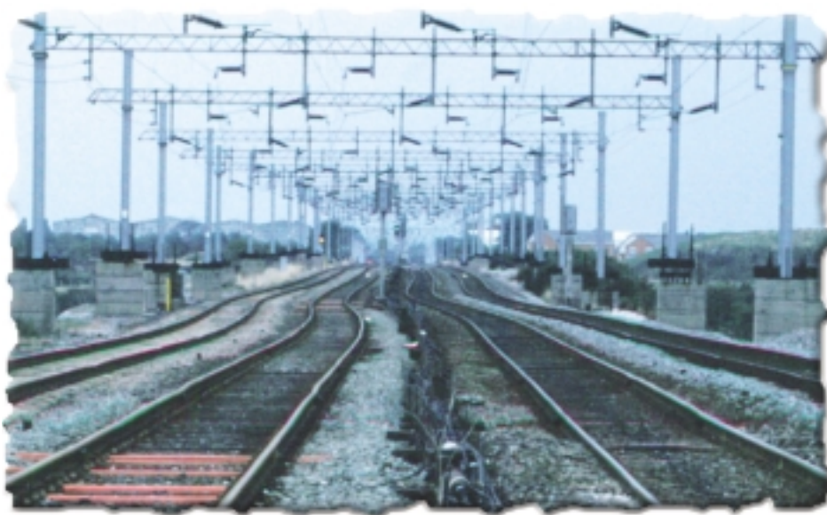
Distorted railway lines over the salt karst (also affected by brine extraction) near Crewe, Cheshire.
